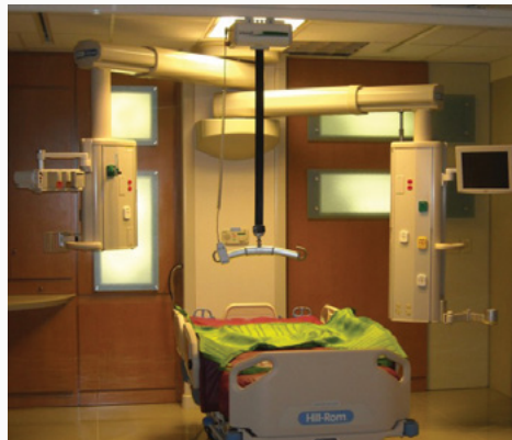
Hillrom-Liko Ceiling-mounted lift in a critical care unit
